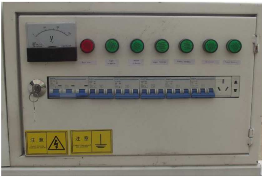
Power control box
